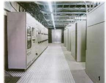
Fixed Ground Power Room 5 x 315 KVA incl. 400 Hz distribution
